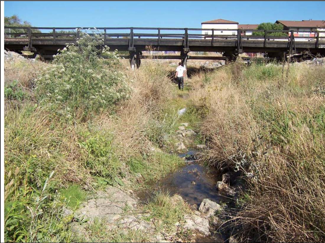
Figure 31. This upstream-facing image shows the railroad trestle running across Wildcat Creek. The railroad trestle acts as a clogging mechanism during the rainy season and traps large woody debris and garbage in the support struts. The significance of this structure as a migration obstacle to salmonids varies depending on the quantity of debris constricting stream flow from year to year.
