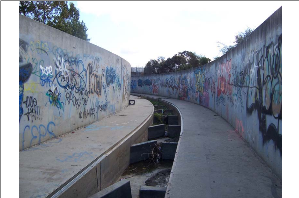
Figure 29. Facing upstream, this photo shows the fish ladder's central conduit and thalweg. The Washington baffles in the thalweg are clearly shown. Some debris is stuck in the baffles. In the rainy season, debris occlusion in the baffles may render the fish ladder thalweg impassable to rainbow trout. Graffiti covers nearly every surface of the structure, which speaks to the fish ladder's highly urbanized setting.
