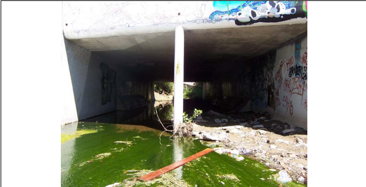
Figure 48. Upstream-facing picture of the Church culvert with graffiti and trash visible in the right conduit.
