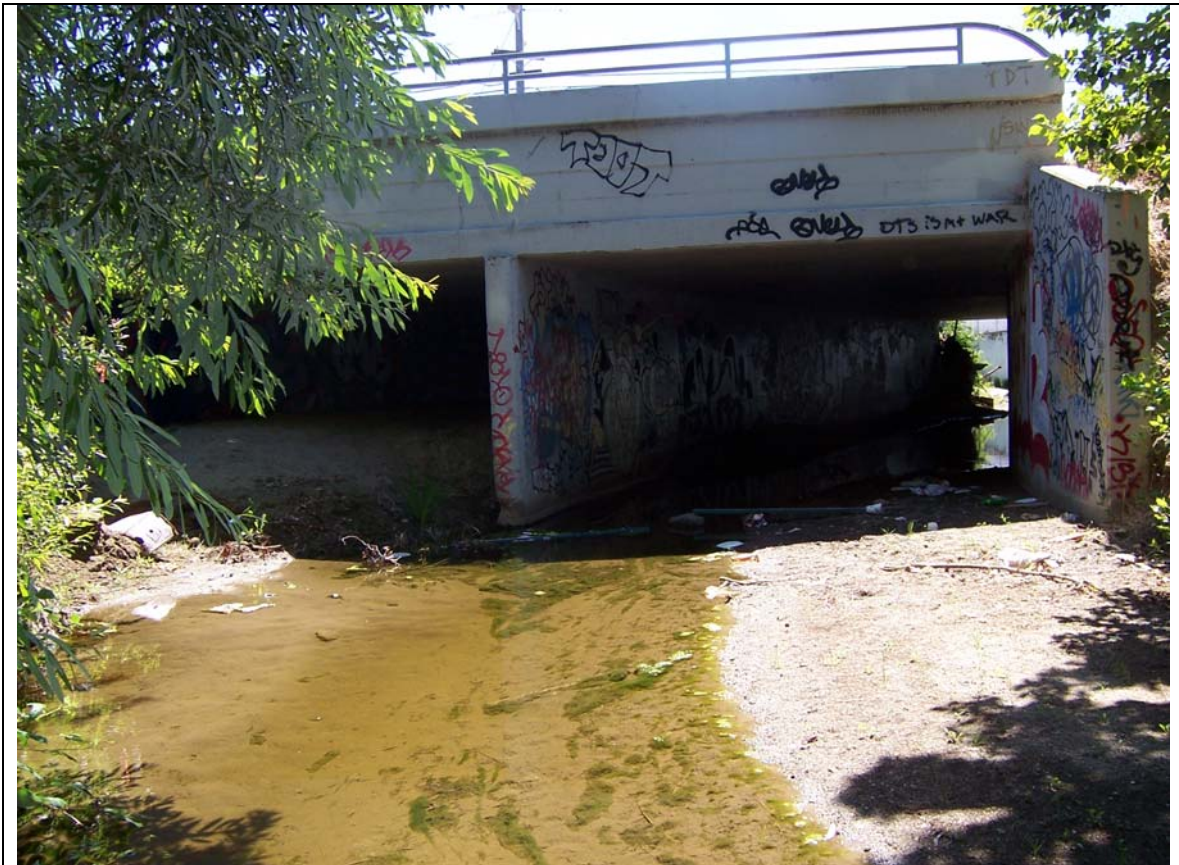
Figure 32. Upstream-facing image of the Rumrill double box culvert with its concrete bottom. Garbage is visible at the base of the culvert.
