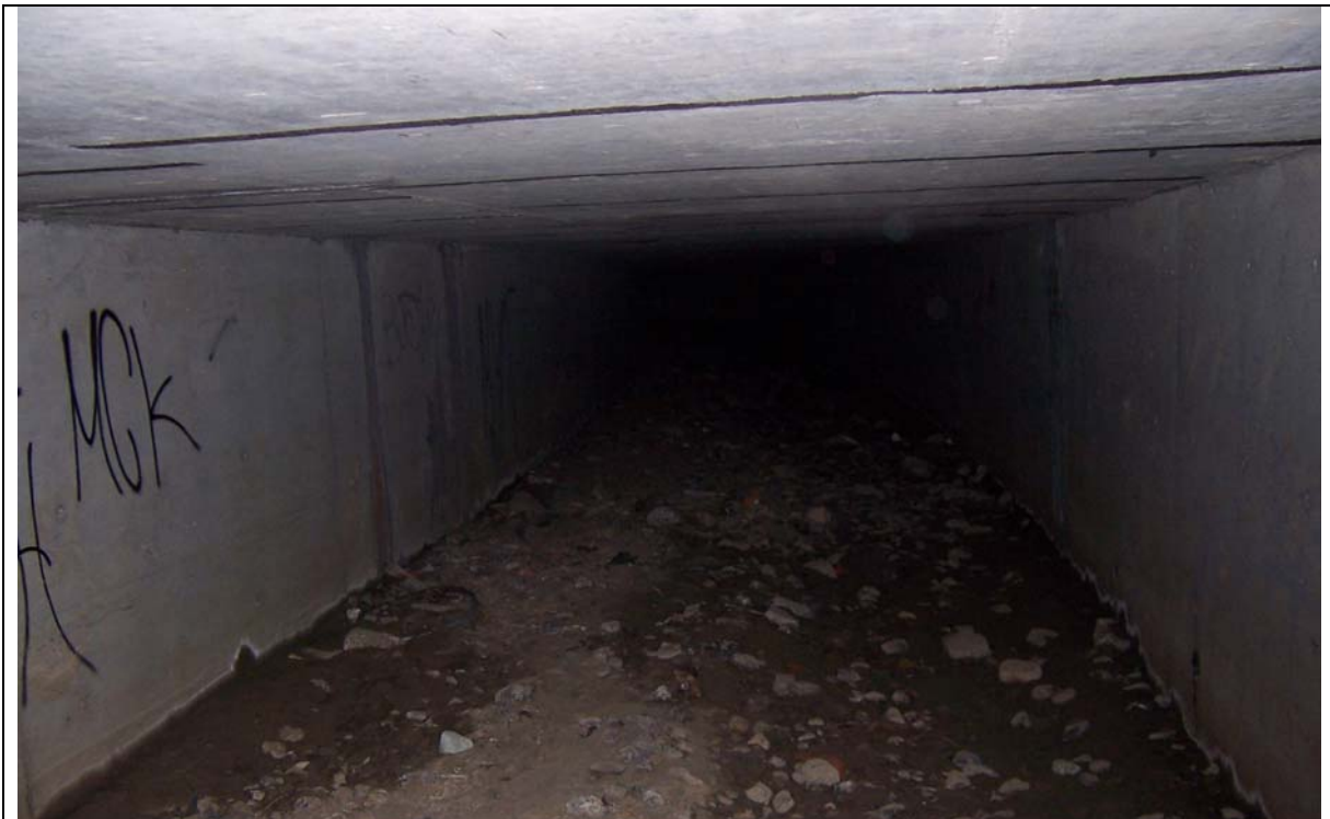
Figure 38. This image was taken 240 feet into the right bank conduit of the Davis Park culvert. The culvert bottom was comprised of sediment of various sizes. The average height at this point was 6' 2". Graffiti was found throughout the culvert.
