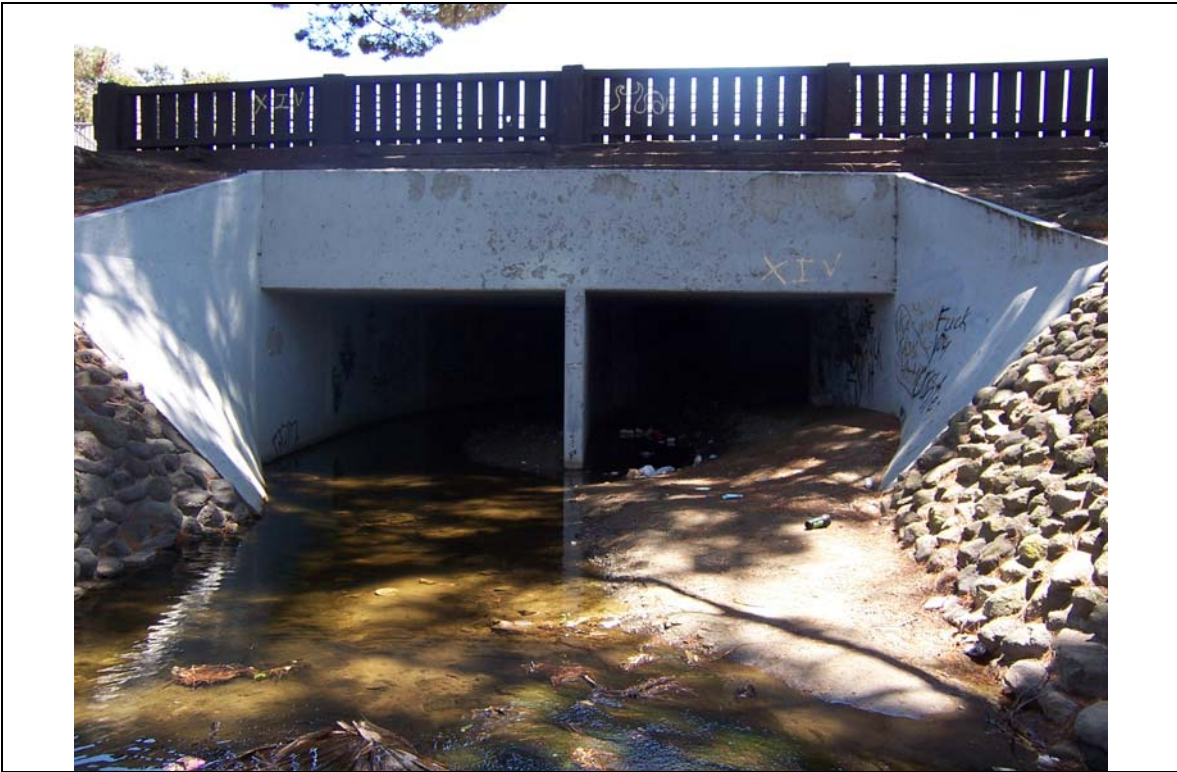
Figure 36. This upstream-facing image shows the Davis Park culvert. Sacrete walls line both the right and left banks and extend outward from the culvert approximately 20 feet.
