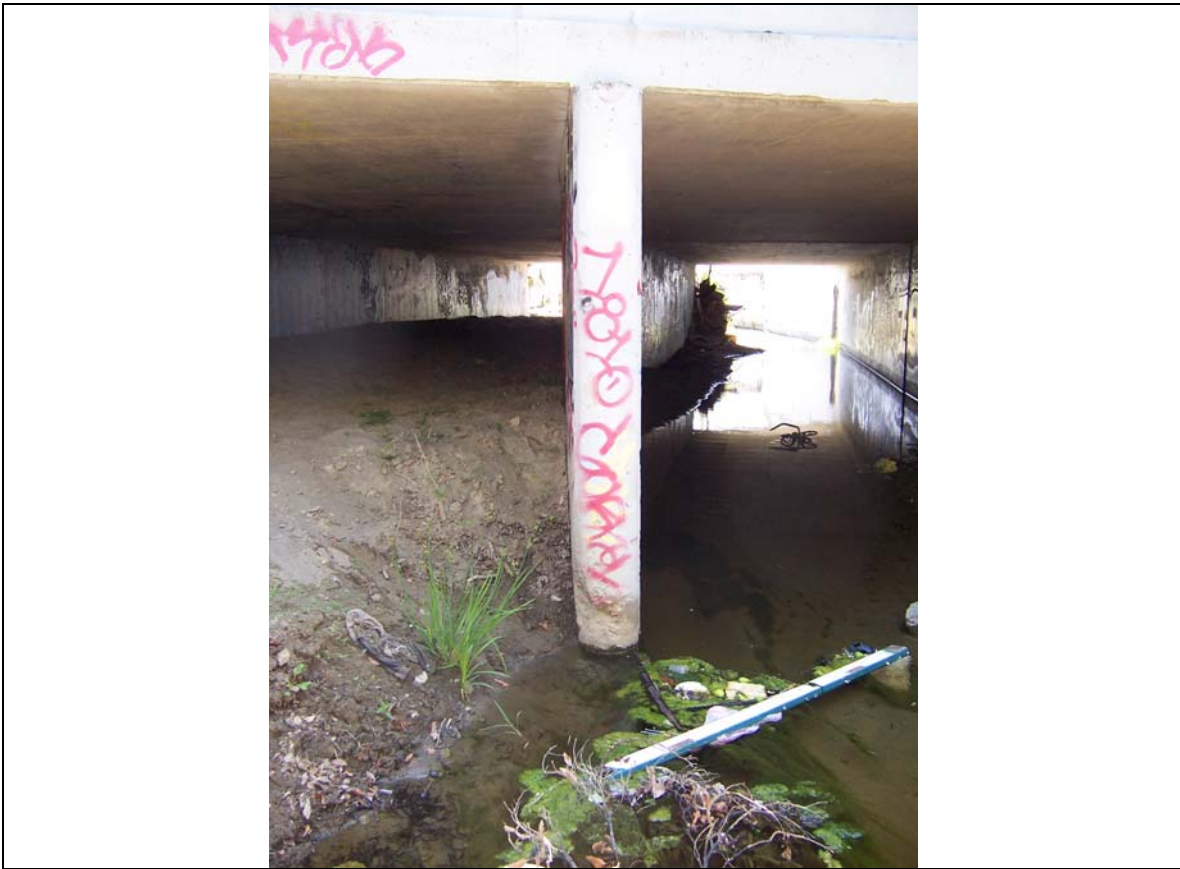
Figure 33. This upstream-facing image conveys the difference in sedimentation between the left and right sides of the Rumrill double box culvert. The left side of the culvert is filled with fine sediment that is approximately four feet and five inches deep.
