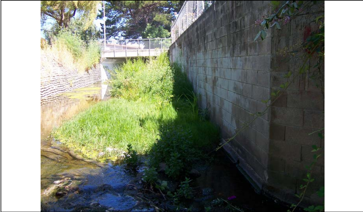
Figure 46. Upstream-facing image of the channel just downstream of the Van Ness culvert.
